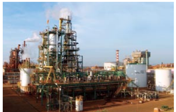
Second phase construction of nickel refining plant for Coral Bay Nickel Corporation, the Philippines
