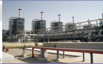
Existing Water & Power facilities (U.A.E.)
